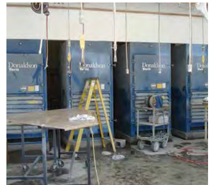
DWS on Granite Finishing 22,000 cfm (37,370 m 3 /h)
