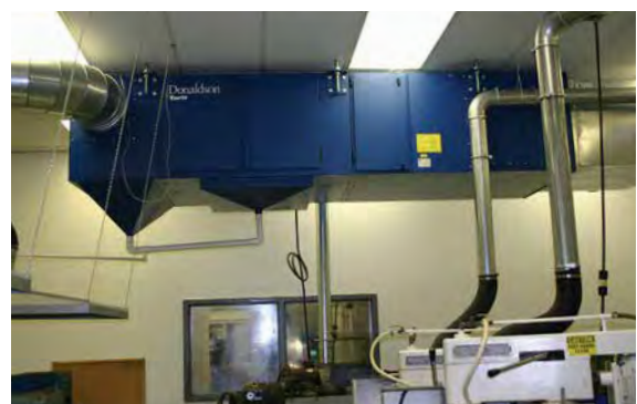
Modular Mediafilter™ on Grinding 2,000 cfm (3,397 m 3 /h)
