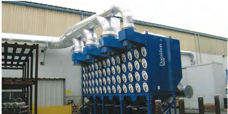
DFO on Grinding 74,000 cfm (125,700 m³/h)
