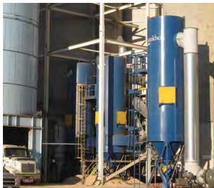
RF - Grain Terminal 34,000 cfm (57,754 m 3 /h)
