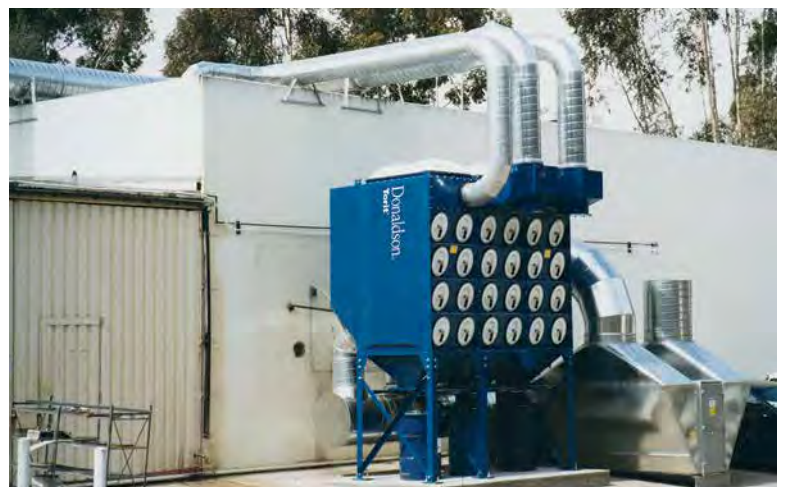
DFO on Metal Grinding 31,000 cfm (52,658 m 3 /h)
