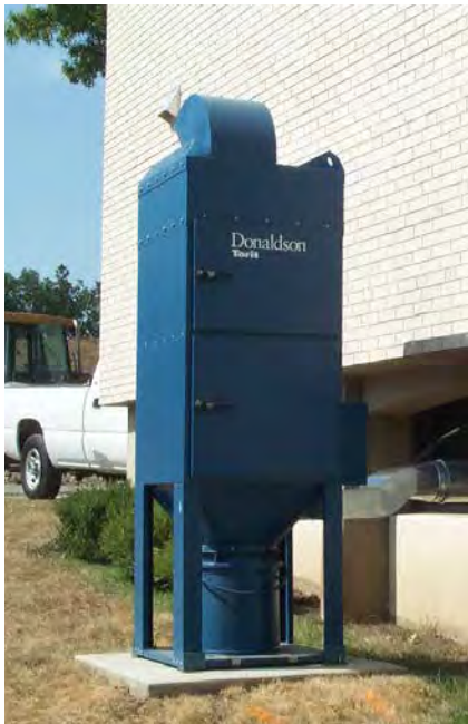
UMA - School Wood Shop 2,000 cfm (3,397 m 3 /h)
