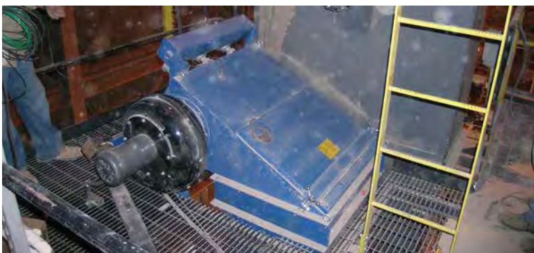
CPV - Bucket Elevator 1,200 cfm (2,038 m³/h)
