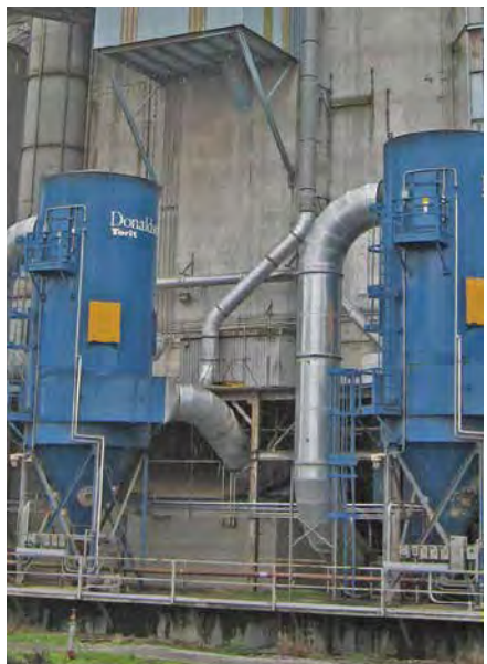
RF - Grain Terminal 61,000 cfm (103,618 m 3 /h)
