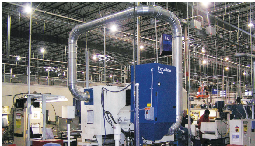
WSO - Machining Center 1,200 cfm (2,038m 3 /h)
